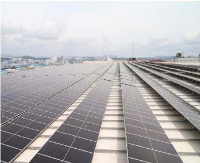
Sihwa MTV Center Solar Power Facility
